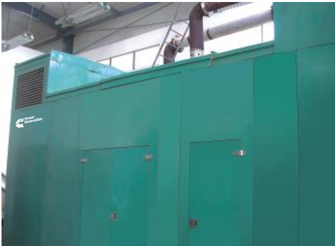
750 kVA Rental Power genset at ITC's plant
