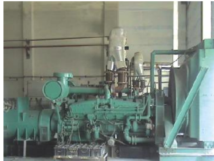
1250 kVA installation at Moser Baer's Photo Voltaic plant
