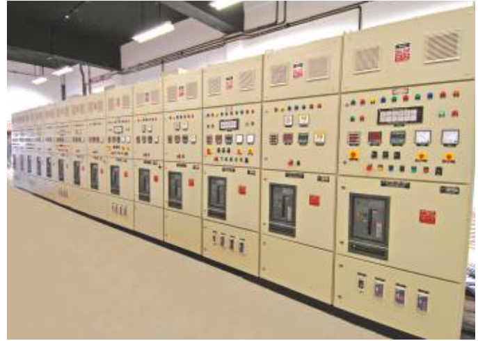
Control panel for the diesel gensets installed on site
