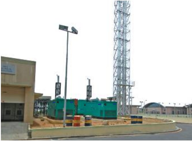
The ICC site features two 500 kVA domestic and three 1010 kVA imported Cummins powered diesel gensets
