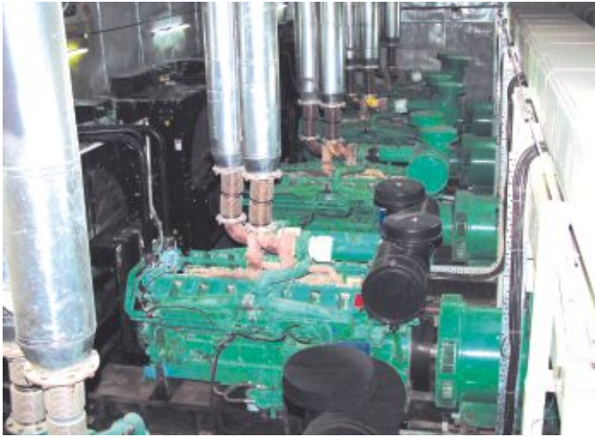
Five 1500 kVA radiator-cooled Cummins gensets inside an acoustically treated DG room
