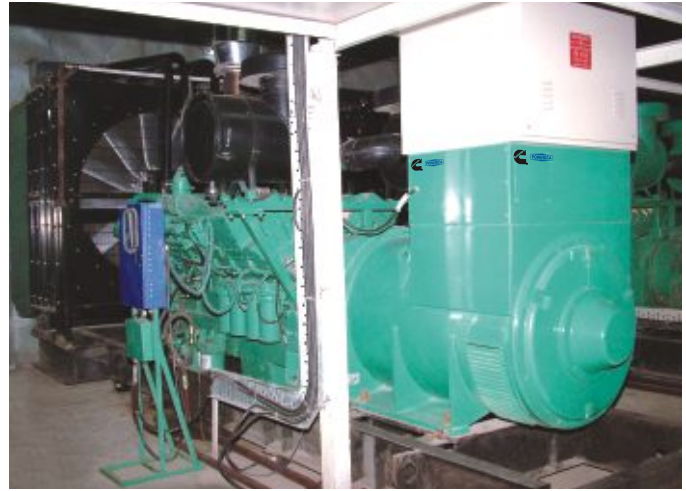
1500 kVA diesel genset manufactured by Cummins
