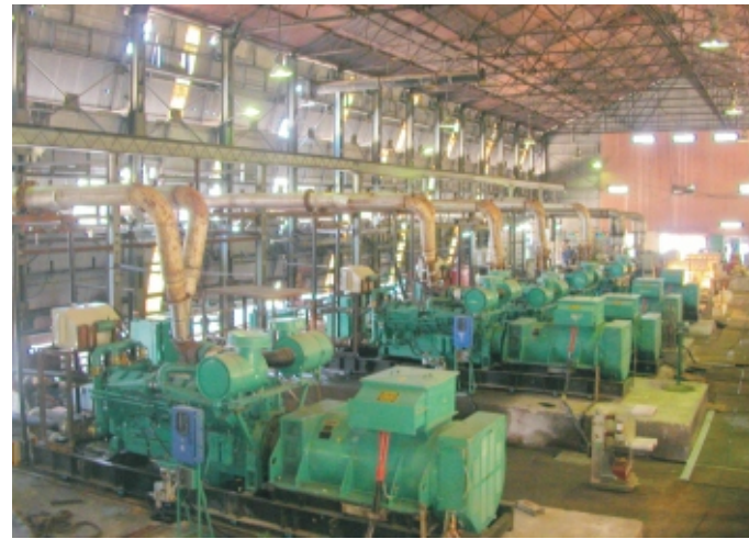
Five 1500 kVA diesel genset - based power plant at Port Blair
