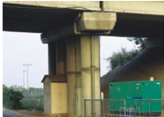
Cummins gensets ensure uninterrupted working of the flyway lighting, toll plaza systems, office systems etc.
