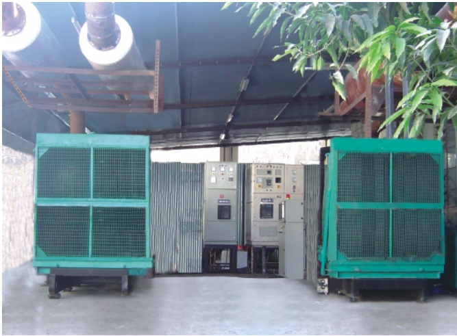
Two 1000 kVA gensets on standby mode for a rental tenure of eight months
