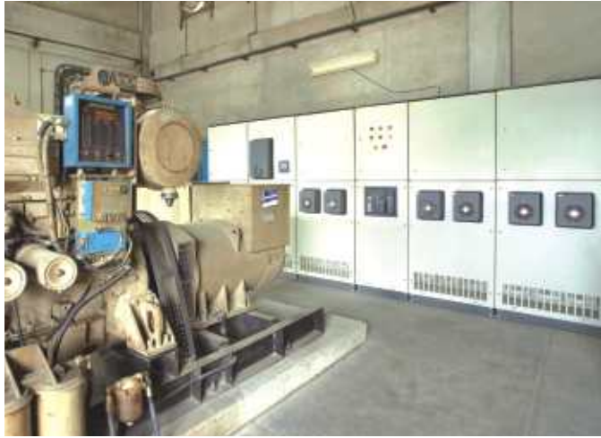
Unbalanced RTPFC cum Harmonic Filtration System (1260 kVAr rating) installed by Cummins Power Generation
