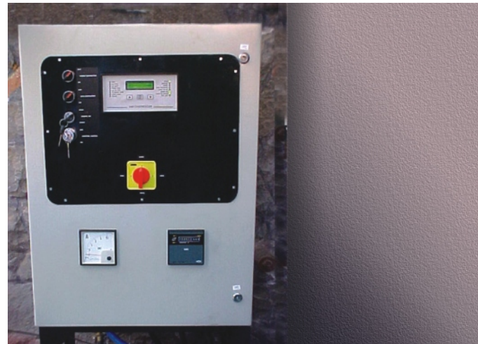
Micro processor based Auto Mains failure panel
