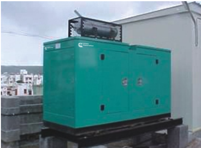
15 kVA acoustically enclosed rooftop installation
