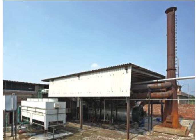
Exhaust Waste Heat Recovery system installed on Cummins gas based power plant to produce steam for the processing plant at K C Fibres Ltd.
