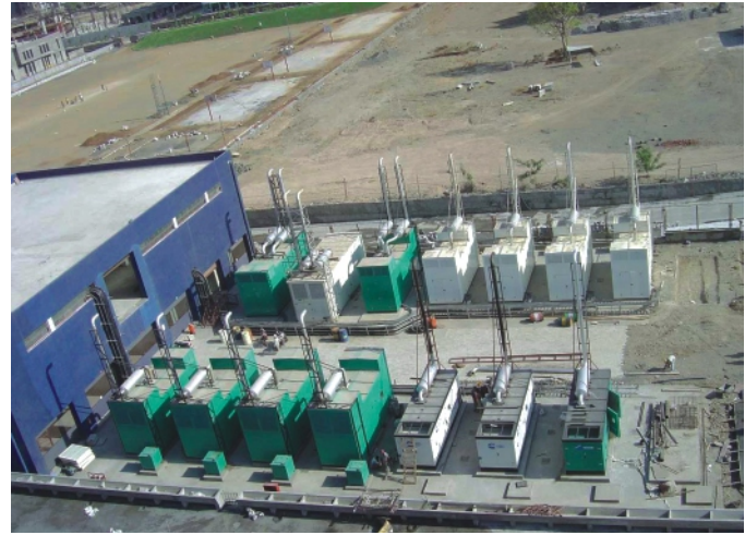
Aerial view of the fourteen Cummins gensets behind Tower III at Magarpatta City
