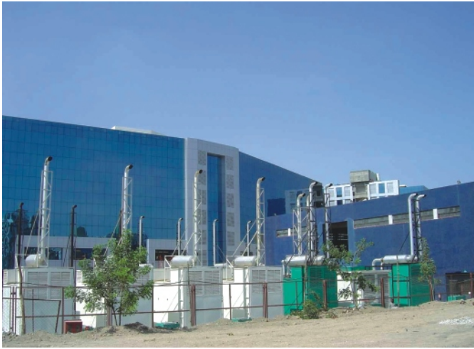
Cummins installations (two 1000 kVA, one 750 kVA & eleven 500 kVA) behind Tower III at Magarpatta City
