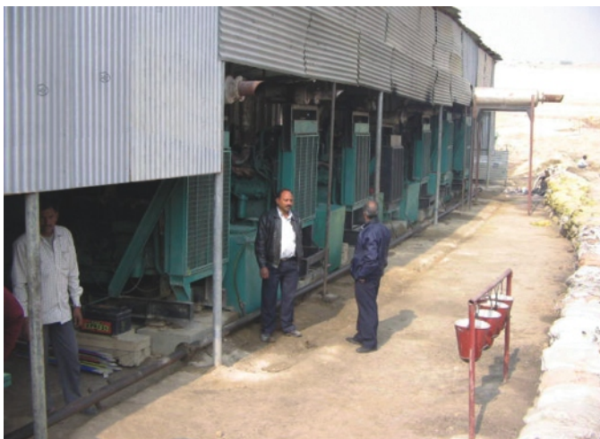
Genset house in the mining pit which is moved depending upon the location of the mining activity
