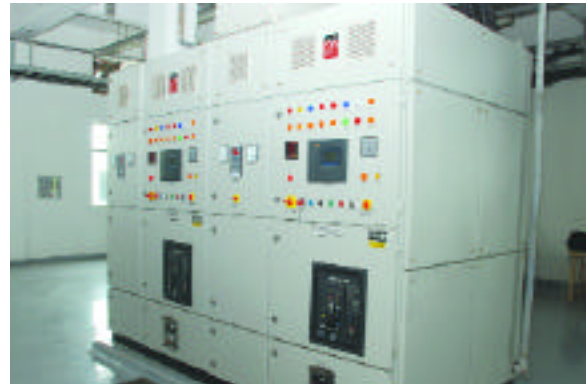
The synchronization panels at the site
