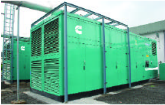
The 2 x 1250 kVA diesel generator sets on duty at Pfizer
