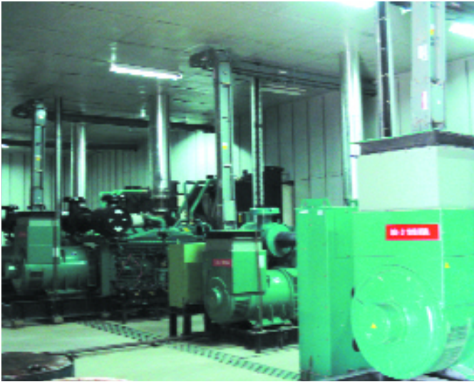
A series of generator sets that provide back-up power to the project
