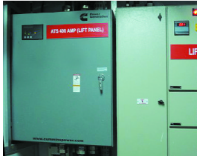
The ATS solution provided by Cummins Power Generation
